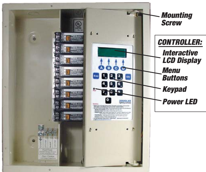
LitePak Panel - Controller Module Mounted
